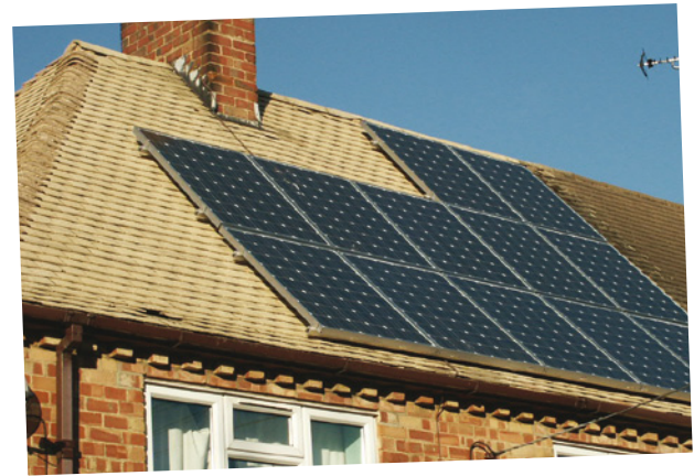
Photovoltaic panels on south facing rear roof
