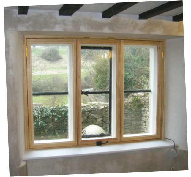
The newly insulated internal walls and secondary glazing, both of which were yet to be painted
