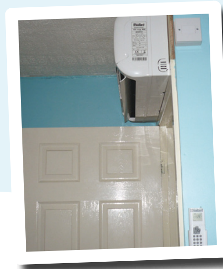
The air source heat pump system is operated with a remote control – seen in a wall mounted cradle.
