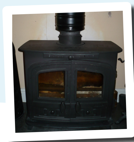
Log burner installed in living room
