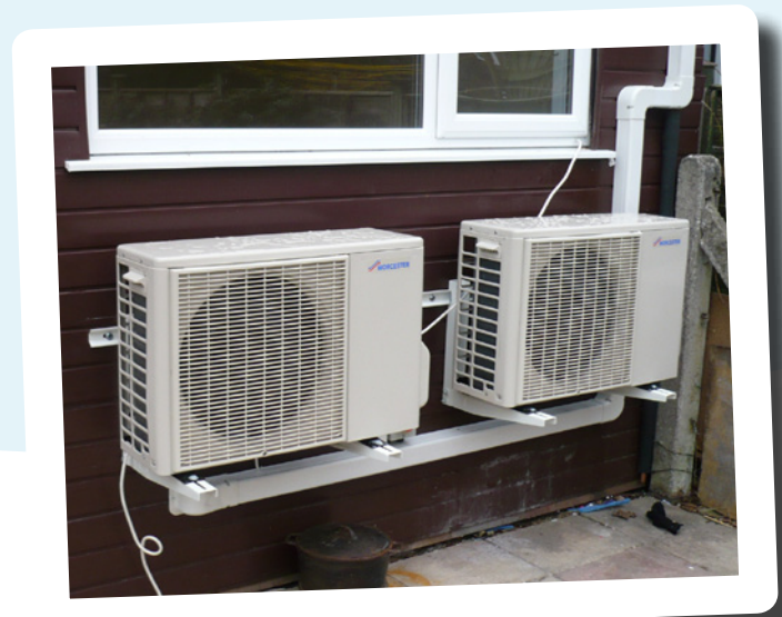
The two air source heat pump units mounted on back wall of house
