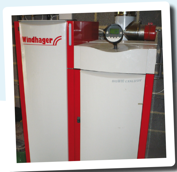
Wood pellet boiler and hopper
