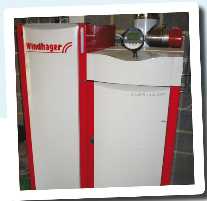
Wood pellet boiler and hopper
