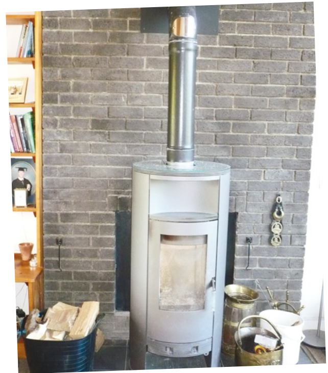
High efficiency woodburning stove
