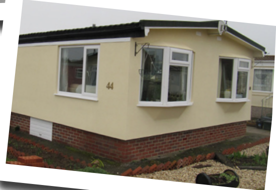
Top: External insulation attached to wall of park home Above: Completed installation, windows are now slightly recessed compared to photo on front page
