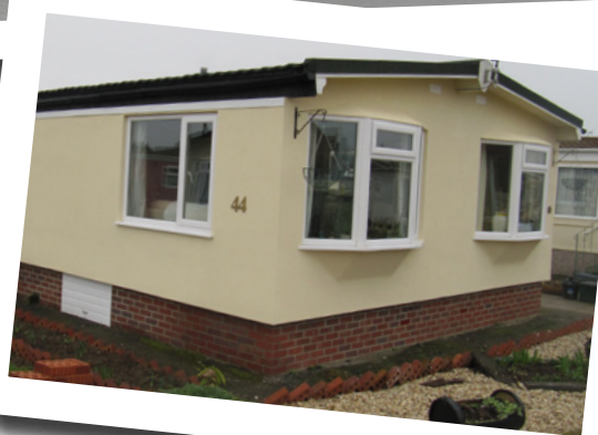
Top: External insulation attached to wall of park home Above: Completed installation, windows are now slightly recessed compared to photo on front page
