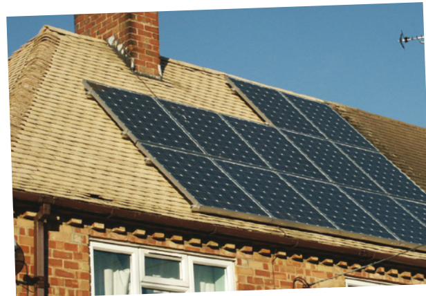
Photovoltaic panels on south facing rear roof
