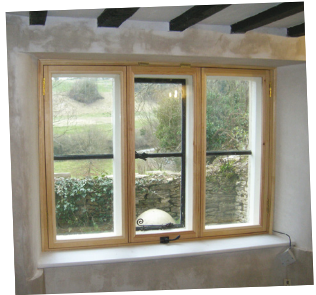
The newly insulated internal walls and secondary glazing, both of which were yet to be painted
