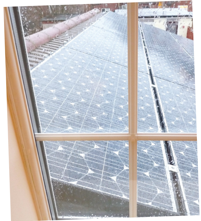
PV system installed on the roof of the extension
