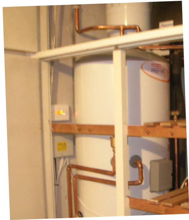
Twin coil hot water cylinder installed in airing cupboard
