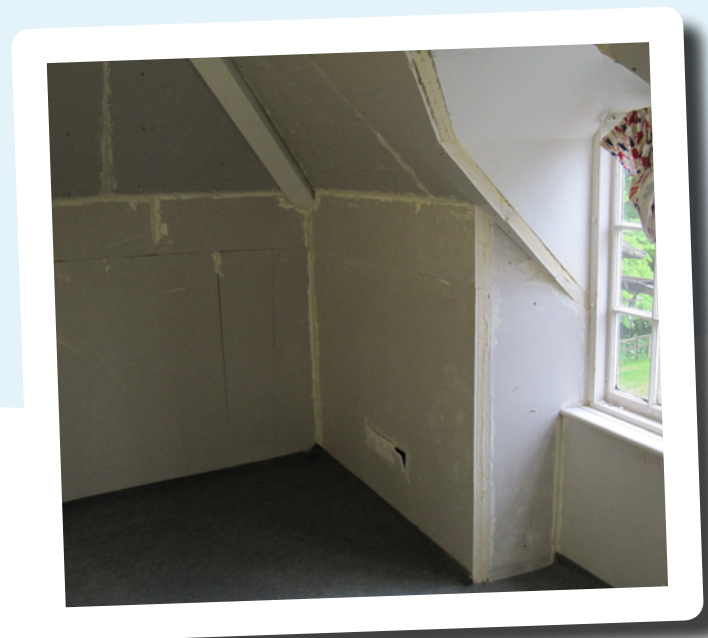
Insulation applied to walls, sloping ceilings and around windows of top floor
