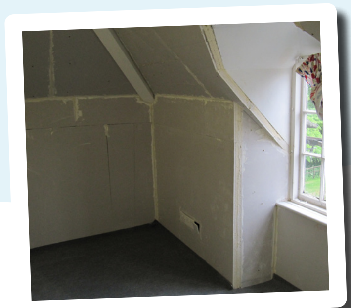
Insulation applied to walls, sloping ceilings and around windows of top floor
