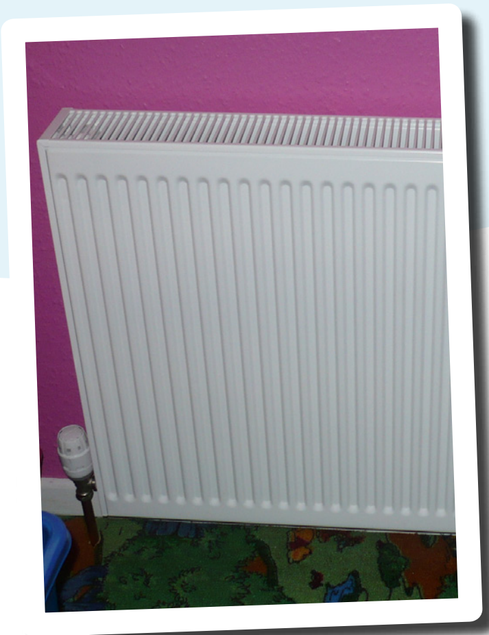
Full central heating installed with radiators in each room
