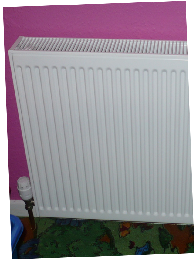
Full central heating installed with radiators in each room
