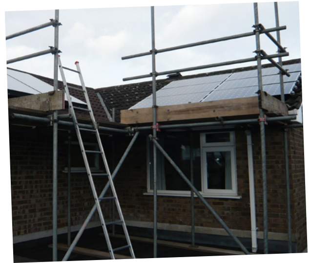
PV and solar thermal panels mounted on south east and south west facing roofs
