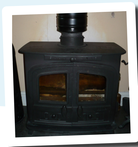
Log burner installed in living room
