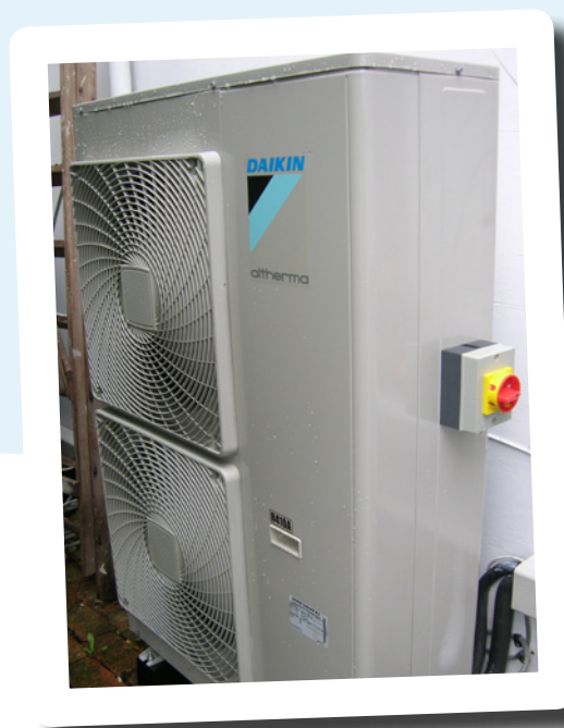
One of the two air source heat pump units installed outside the house
