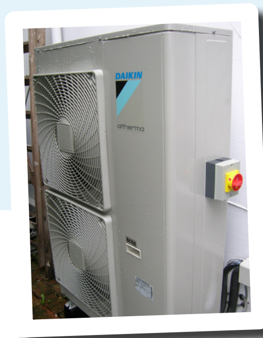
One of the two air source heat pump units installed outside the house
